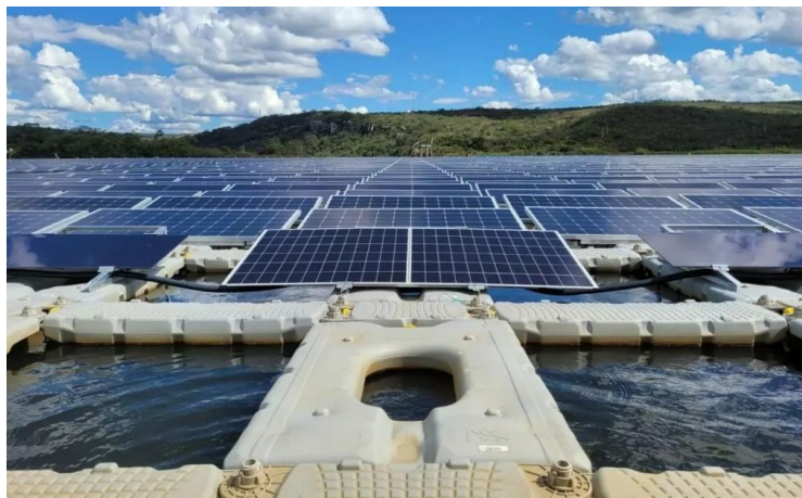
Fig. 2: Solar photovoltaic station installed on the surface of a natural hydro accumulative electric station reservoir.
